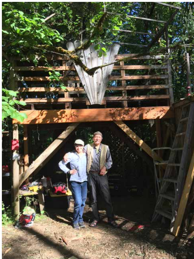
Jim and Rose doing booth construction in 2023. Peter made the sunburst several years ago, these guys made a window in it and shored up the floor.
